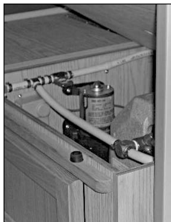
Picture G-P17: Water heater access door.
